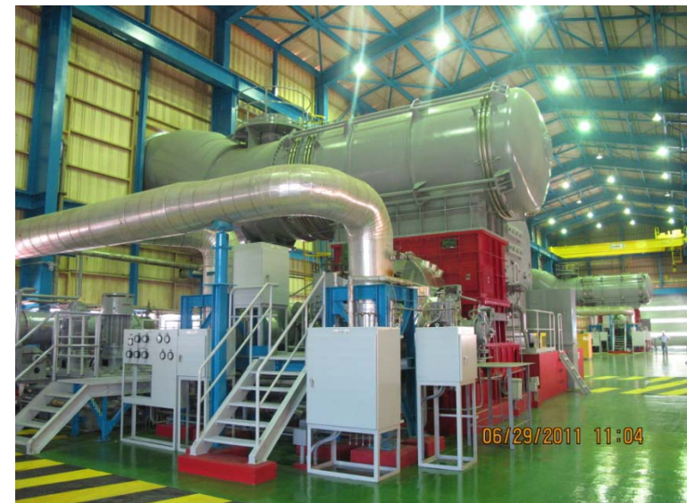
Makban Plant E
