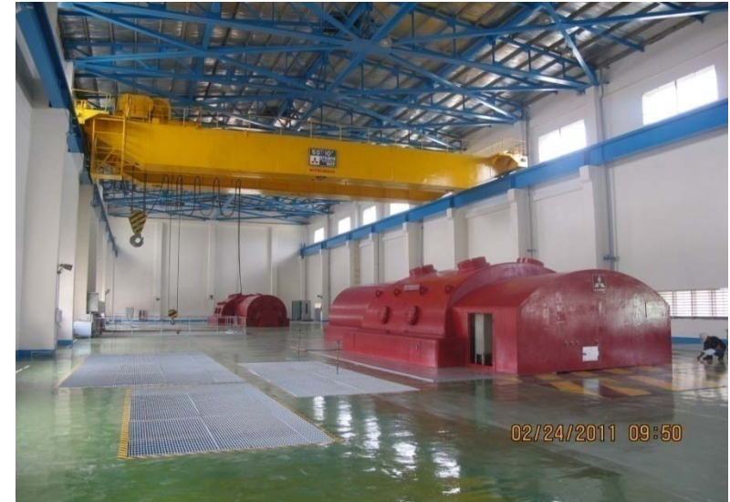
Makban Plant A
