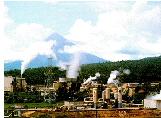
Tiwi Geothermal Power Plant Complex
