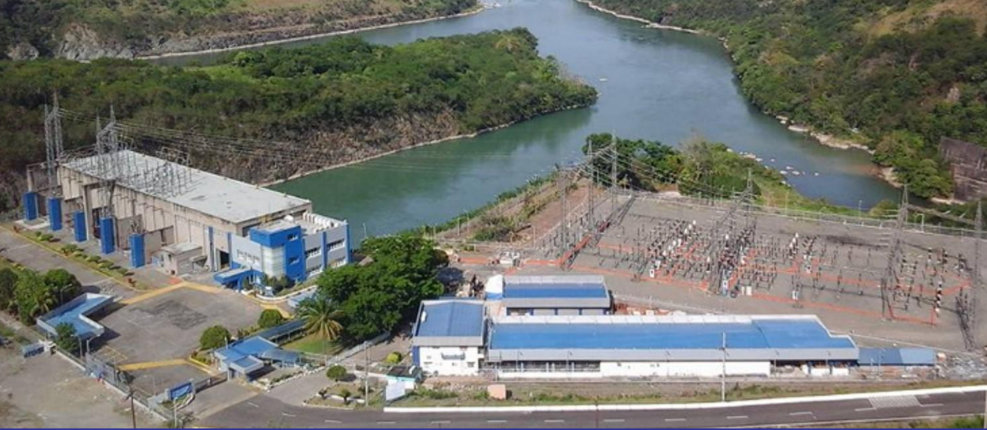
SNAP Magat Battery Energy Storage System (BESS) 20 MW
