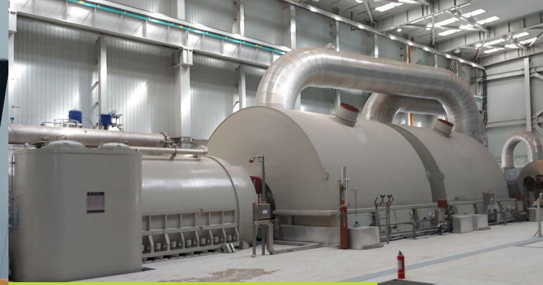
Unit 1 Steam Turbine Generator
