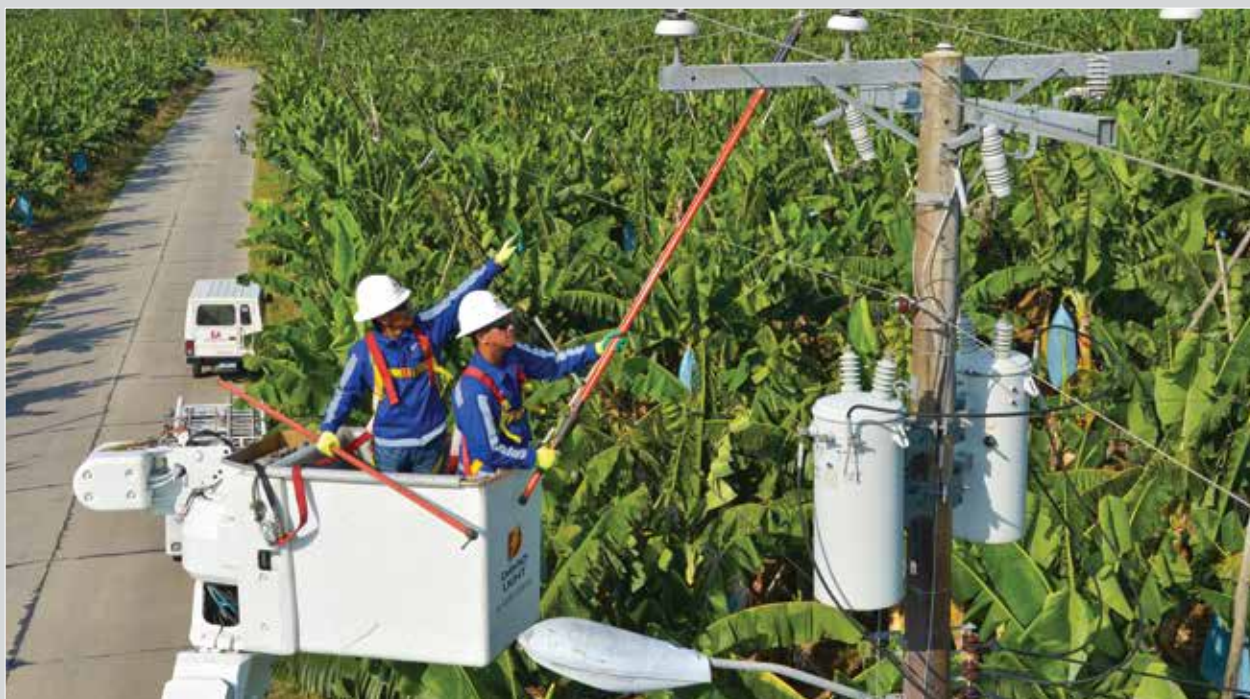
The Distribution Business Group prepares for the future by building more infrastructure in its distribution and sub-transmission networks to ensure even more robust, reliable, and flexible systems.
