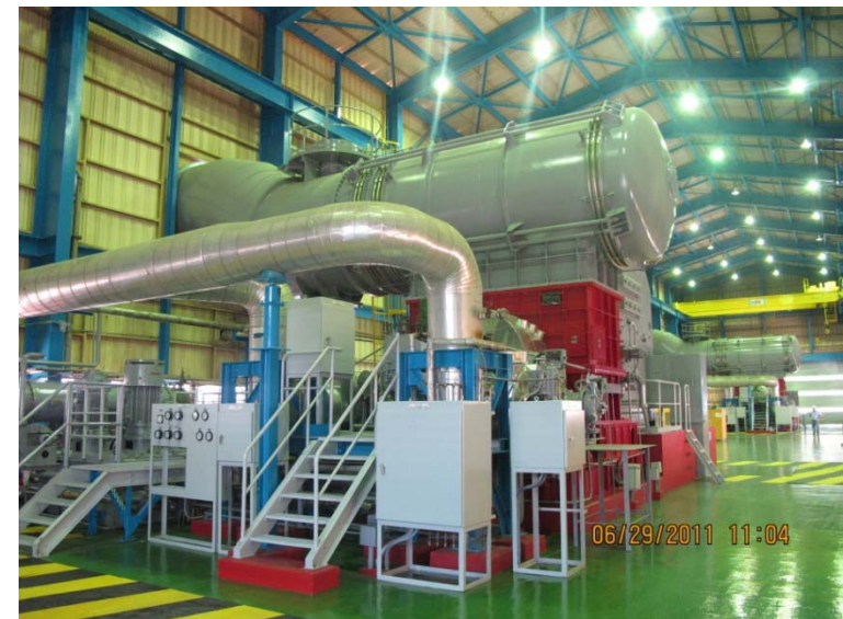
Makban Plant E
