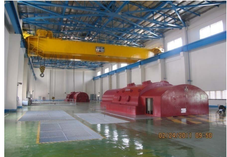
Makban Plant A
